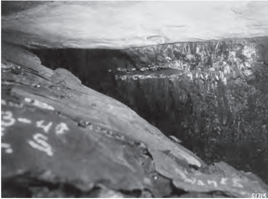
Showing roof fall after explosion.
