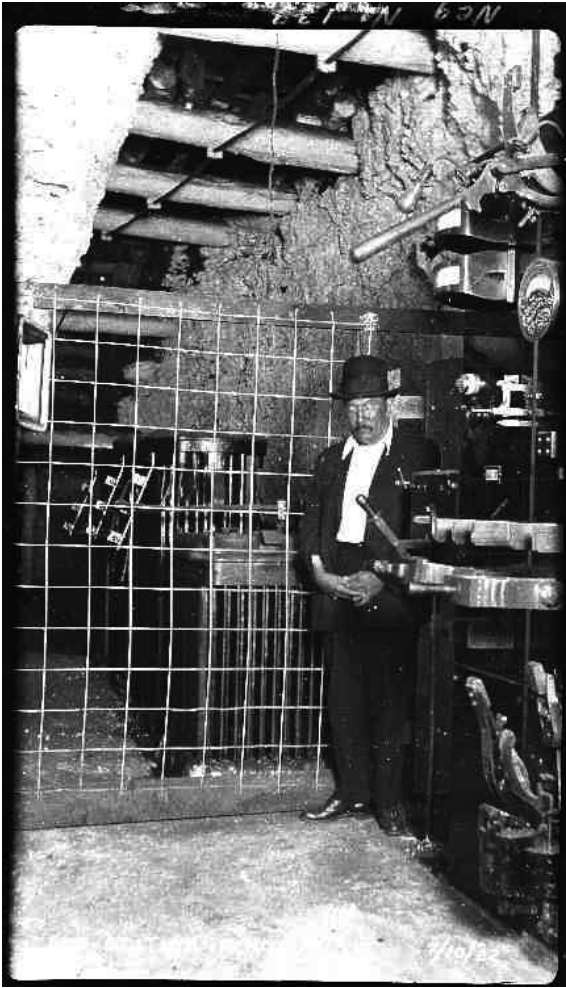
A man minds the substation at the No. 6 Stag Canyon Mine. Photo Courtesy of New Mexico State University Archives.
