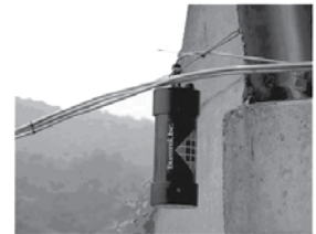
Radio Repeater At Portal
