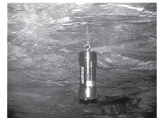
Radio Repeater Underground
