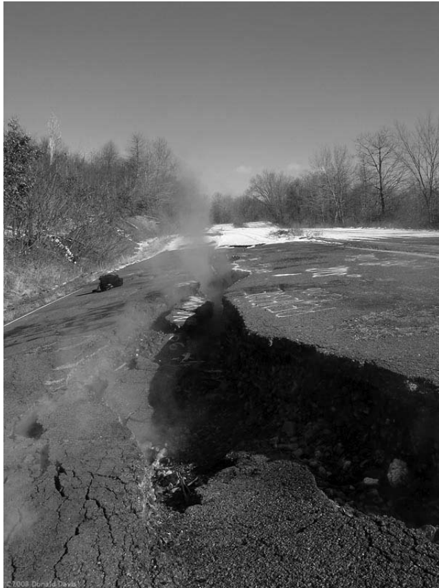
Steam rises from a split in the asphalt along the stretch of Pennsylvania State Highway 61 South of Centralia.
