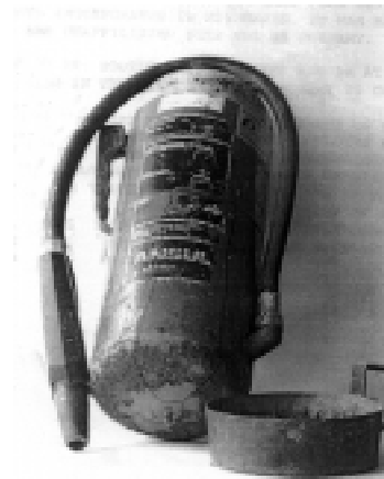
Look at the bottom of the extinguisher for corrosion. Moisture can be trapped inside the rubber base. BE CAREFUL!!!
