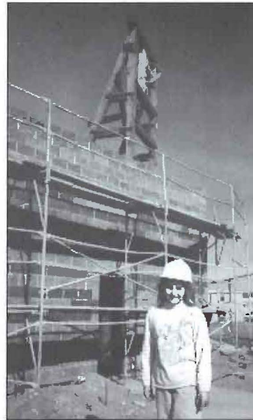
Students of the McCaw elementary school in Henderson, Nev., pose in front of the partially completed "School of Mines"—the first of its kind in the country. Note the headframe in the background.
