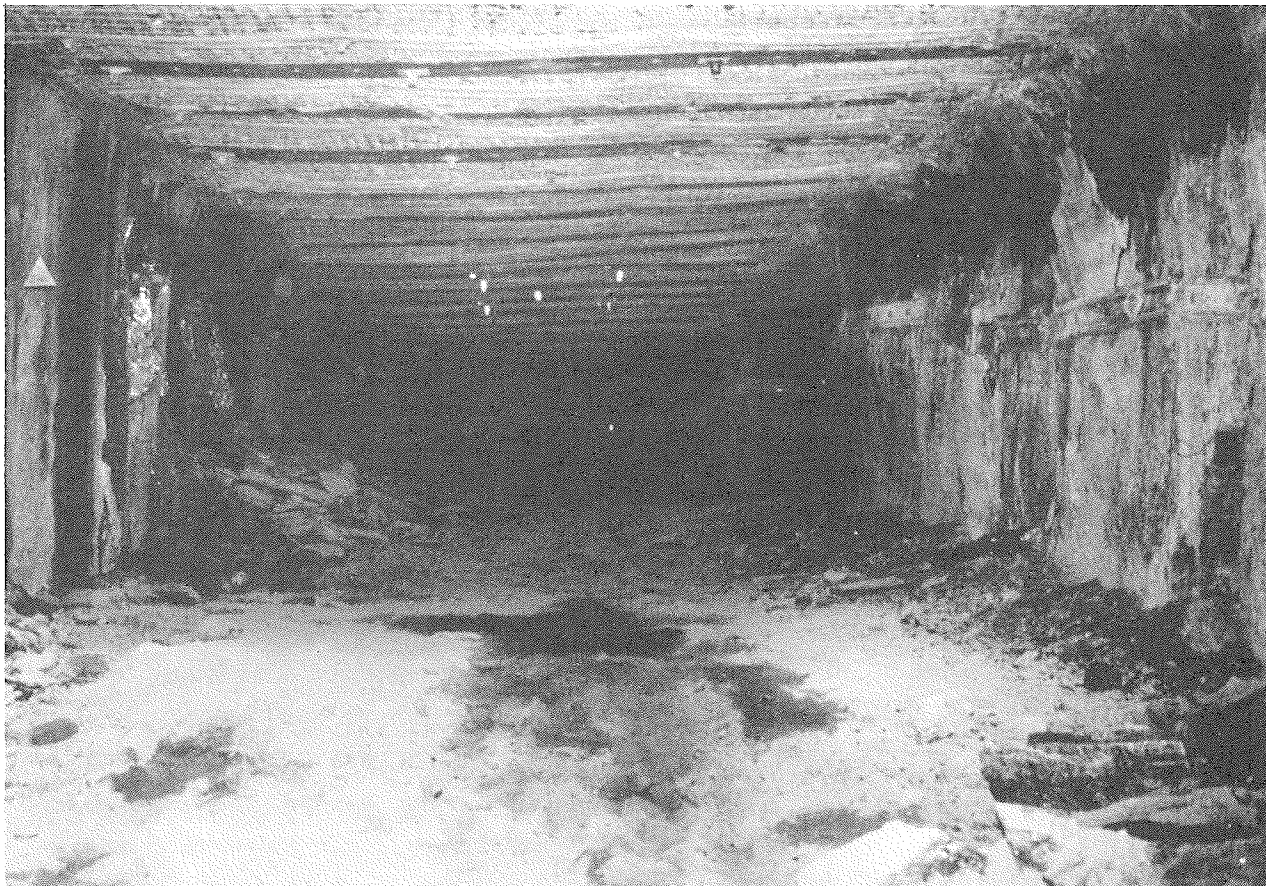
Actual tailgate entry supported with resin-grouted cables subjected to first panel loading.
