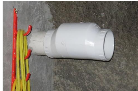
PVC Check Valve in NIOSH BIP
