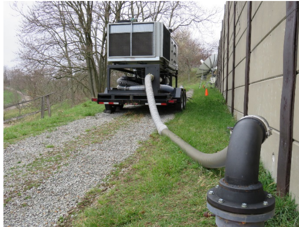
ChemBio Borehole Air Supply
